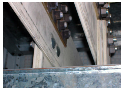
Images Courtesy of HSB Thermography Service
