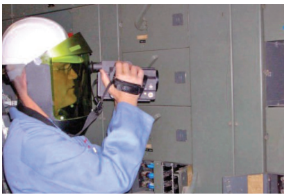
Infrared thermographers look for hot spots that could indicate loose connections and other electrical problems.
