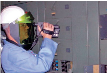
Infrared thermographers look for hot spots that could indicate loose connections and other electrical problems.
