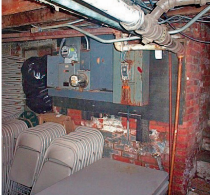
Electrical equipment rooms used for storage create property and liability exposures.
