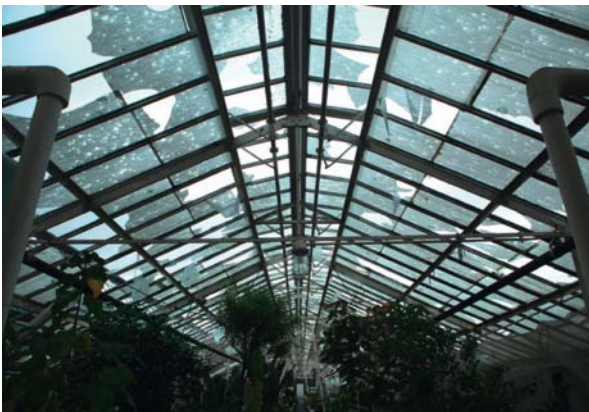
Hail, a by-product of severe thunderstorms, can cause significant property damage.
