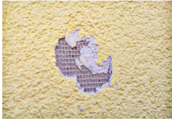
Newer, well-insulated façades with a thin finishing coat proved to be very susceptible to hail damage.
