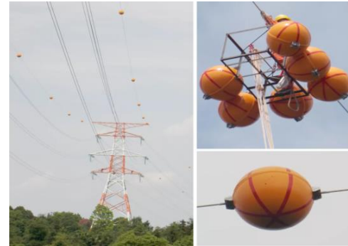
Power Line Marker
