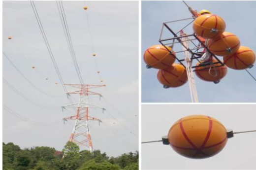
Power Line Marker
