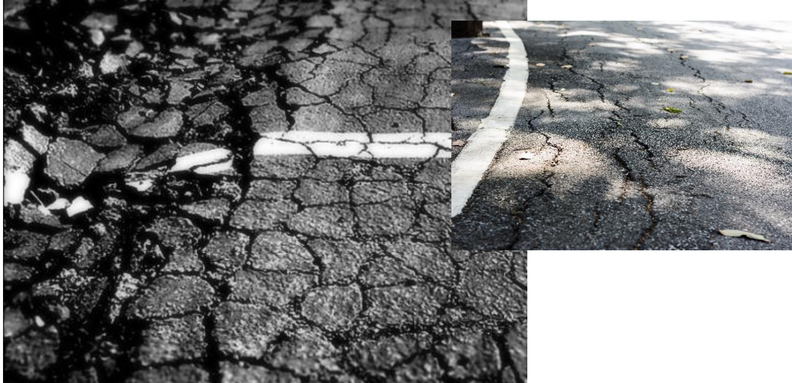
Source: Cracked black asphalt road
