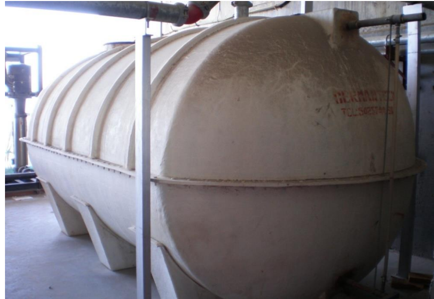
Source : Temporary water tank
