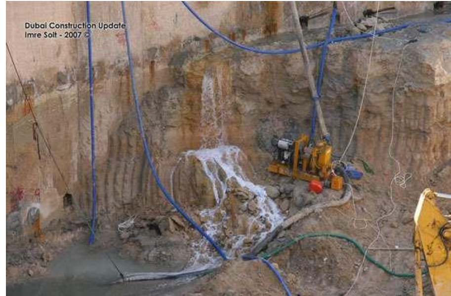
Source: Dubia construction leak
