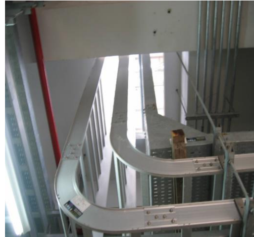
Source: Cable ducts
