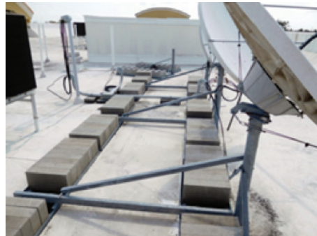
Satellite trays with concrete block ballasts
