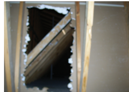
“Unapproved” opening in a draftstop wall.
