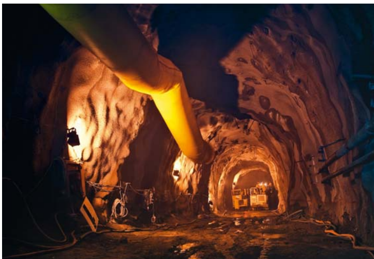
Keeping the Gautrain project on track: The prestigious high-speed rail link between Pretoria and Johannesburg is not just a colossal technological feat. It also presents many challenges for managing the structural and civil engineering risks involved.
